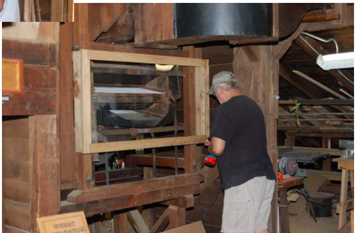
Jerry Kieth is installing the safety cover over the front of the separator.
