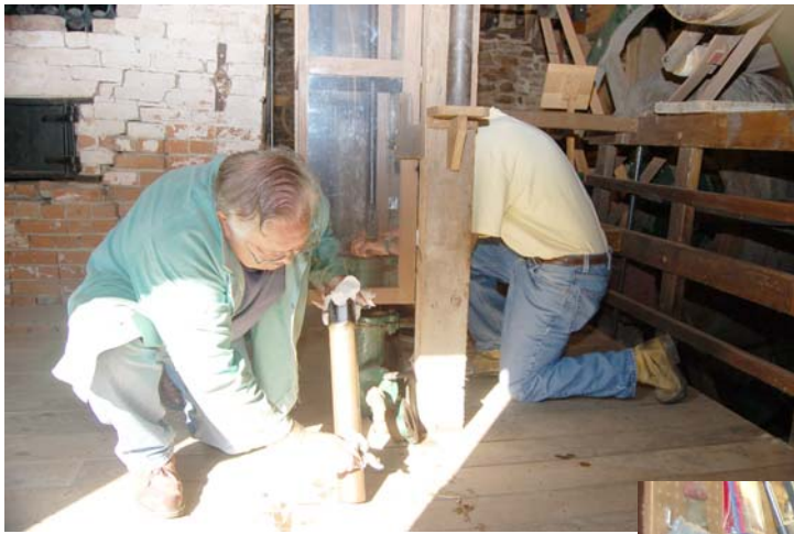
Peter Allenger and Scott Gibbs are working on the stubborn boiler feed pump. Peter is cleaning the piston while Scott checks the valves.
