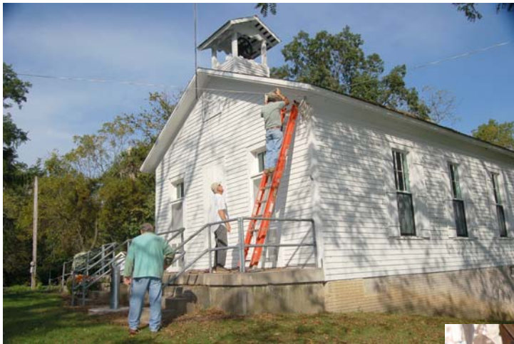
Peter Allenger and Scott Gibbs are stringing the cable and installing the PA speakers for Heritage Day.
