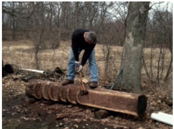
A modern day reenactment of squaring off a hard wood log just as Nye's workers did it.
