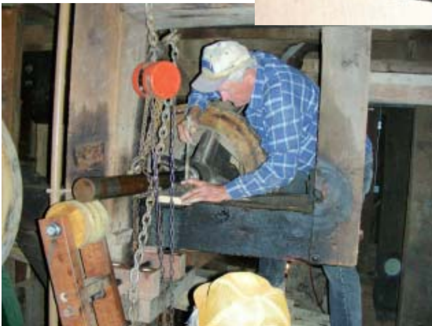
Joe Clark and Peter Allenger are shimming up the south end of the main line shaft in the basement. The hard wood block they are placing under the pillow block raised the shaft to level it.
