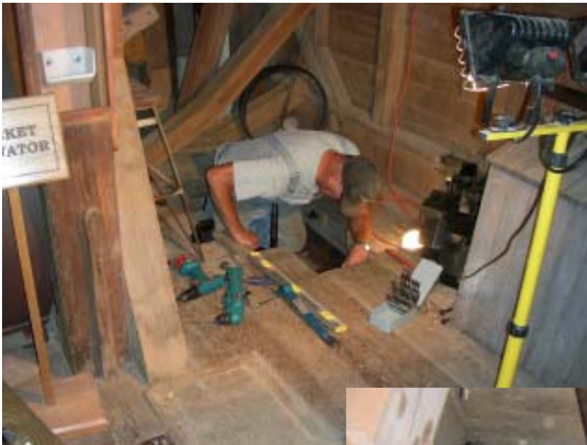
No, Dick Clevenger is not jumping through a hole in the floor. Actually he is standing on the top of the smutter while installing part of the agitator drum. The smutter hangs from the basement ceiling with part of it projecting up into the first floor.
