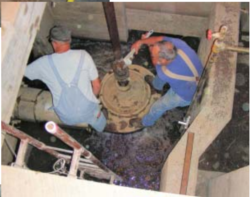
To get ready for Heritage Day Bob Delong and Dick Clevenger are clearing the turbine of mud and getting it turning again. This requires opening up the penstock gate and giving the turbine shaft a few turns with a large pipe wrench to get it moving again. Note the water boiling out from the bottom of the turbine.
